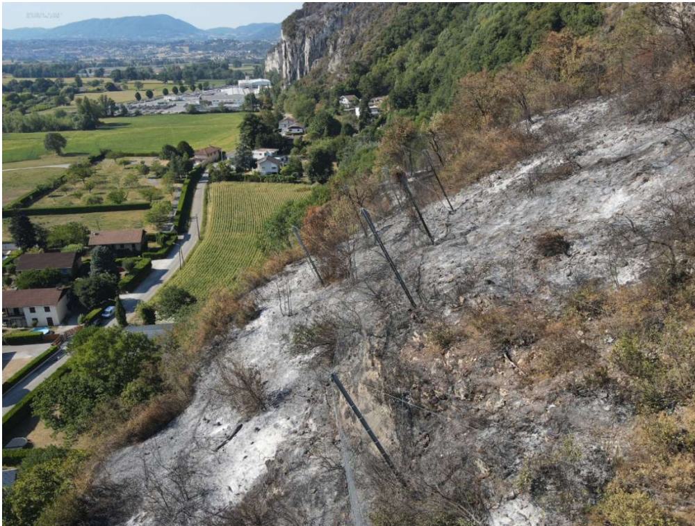
Figure 8 : View of the Balmes structures; northern section (flexible barriers) upstream of the built-up areas. In the background, the hamlet of Le Bourget, which was not affected by the fire. (Source: SDIS 38 – 9 August 2022)
